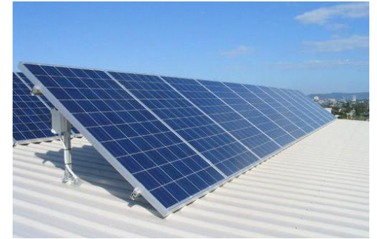
PV rooftop system
